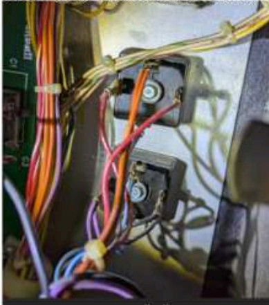
Bridge Rectifiers located in the back box
